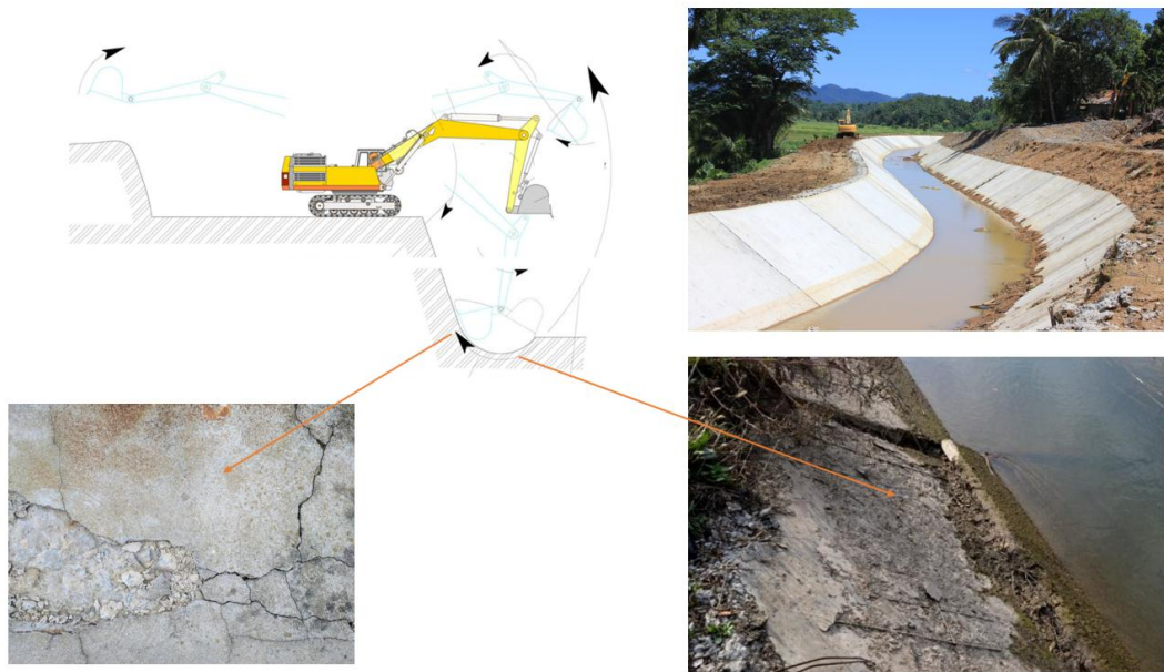
Figure 2. Image of damage to concrete lining from silting of canals.
